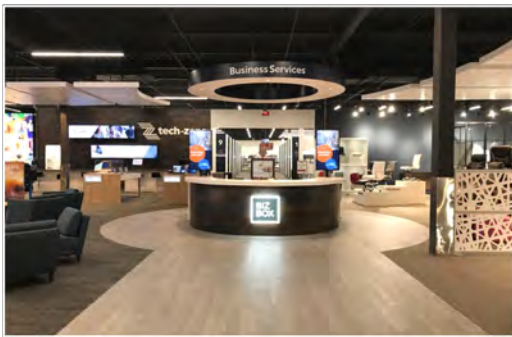
Front Entrance Apollo assisted with the install of the front entrance and business center
